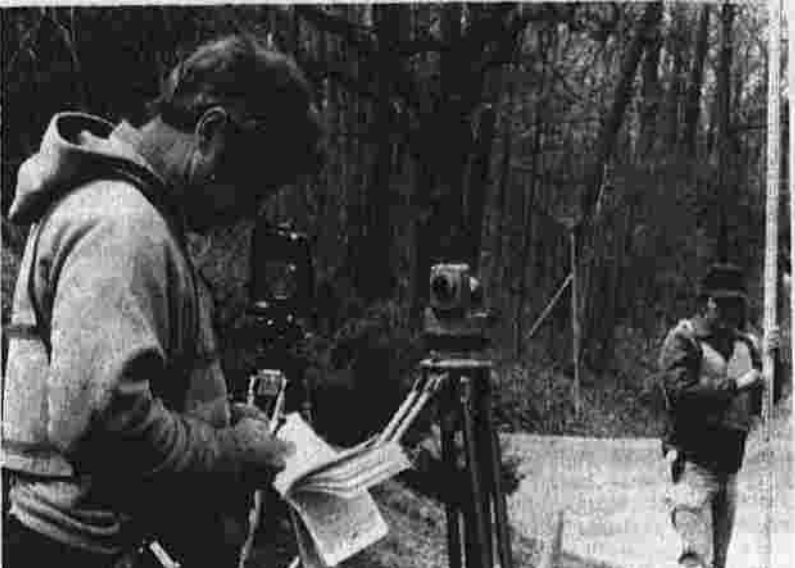
Robert Howarth, left, and Douglas MacGillibray, surveyors, for Fuss and O'Neill, do survey work on Highland Street, Manchester, as part of a town water improvement project. (Herald photo by Pinto)
